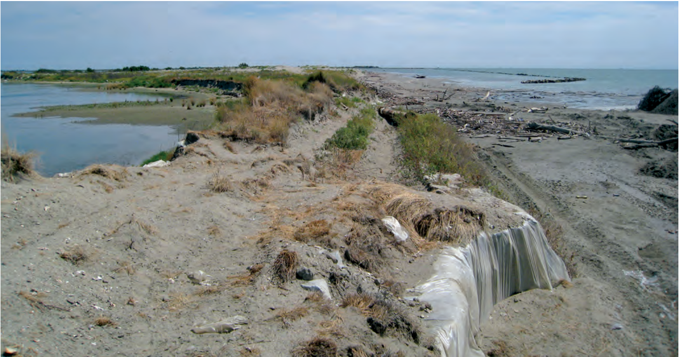
Figure 4: in the foreground one can clearly see the small earthy diaphragm, with its plastic film reinforcement introduced during construction separating the beach from the lagoon, covered with sparse ruderal vegetation. On the lagoon side (left), the presence of intertidal transition surfaces can be noted. This photo dates back to 2009; the sea facing artificial beach is now much larger as a result of recent ebb flow (photo: Bonometto 2009).
